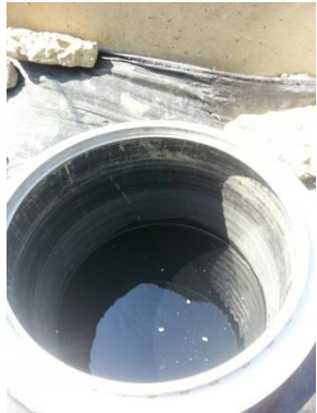
Excessively high water table
